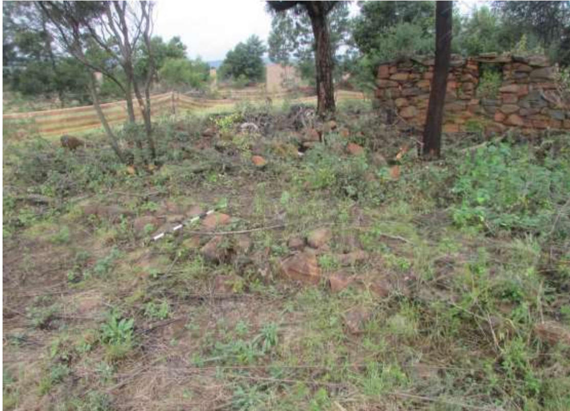
Figure 19: A view of the outside veranda/garden terrace walling at one of the structures.
