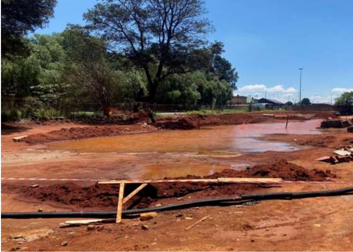
Figure 5: General view of the site in January 2022. Heavy & constant rains over the December/January period caused some damage to the site.
