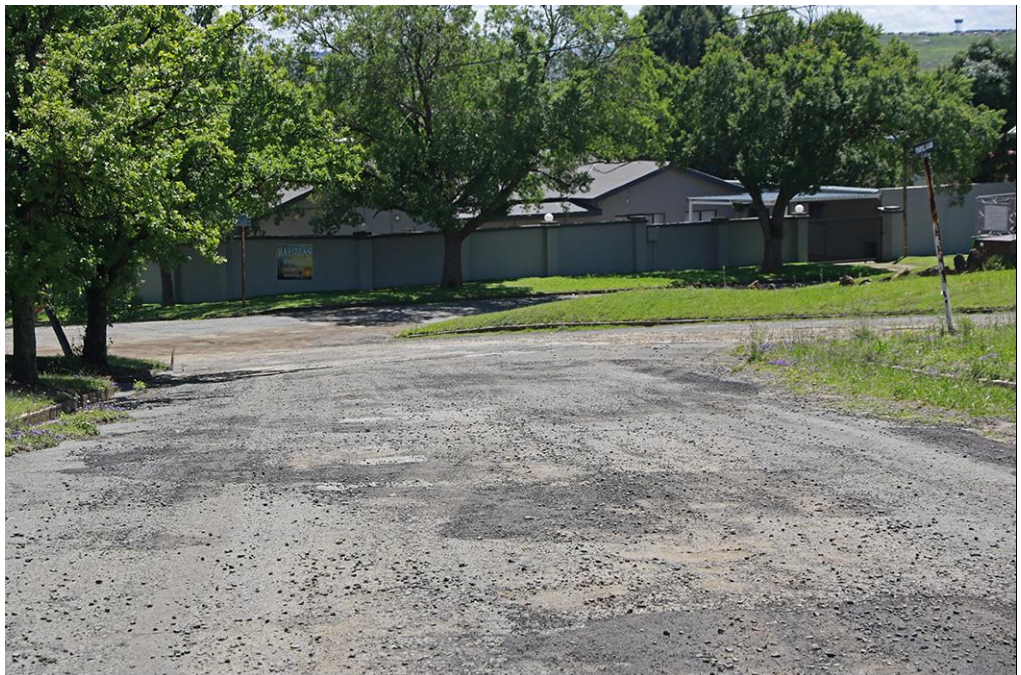
Photo 9: Poor condition of Wilson Street / President Street Intersection
