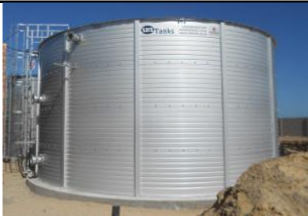
Rainwater storage tank
