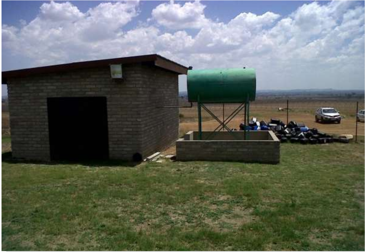
Figure 6: Backup generator and bunded diesel storage tank
