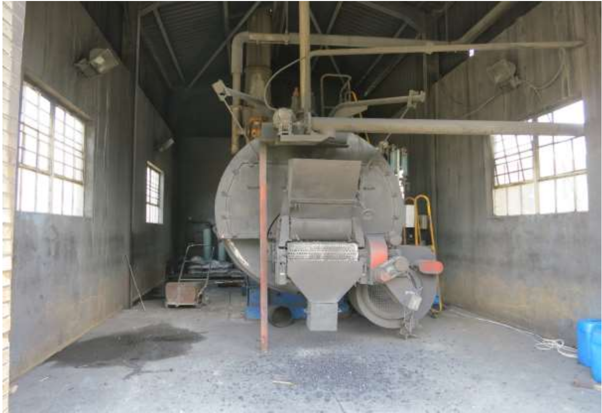
Figure 8: One of two coal fired boilers used to generate steam on site
