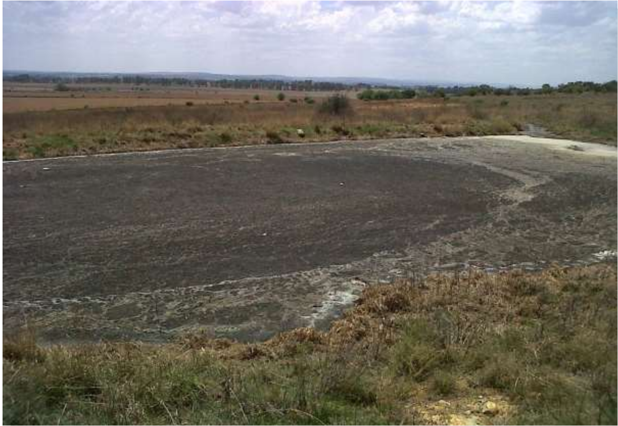
Figure 18: The existing wastewater evaporation pond
