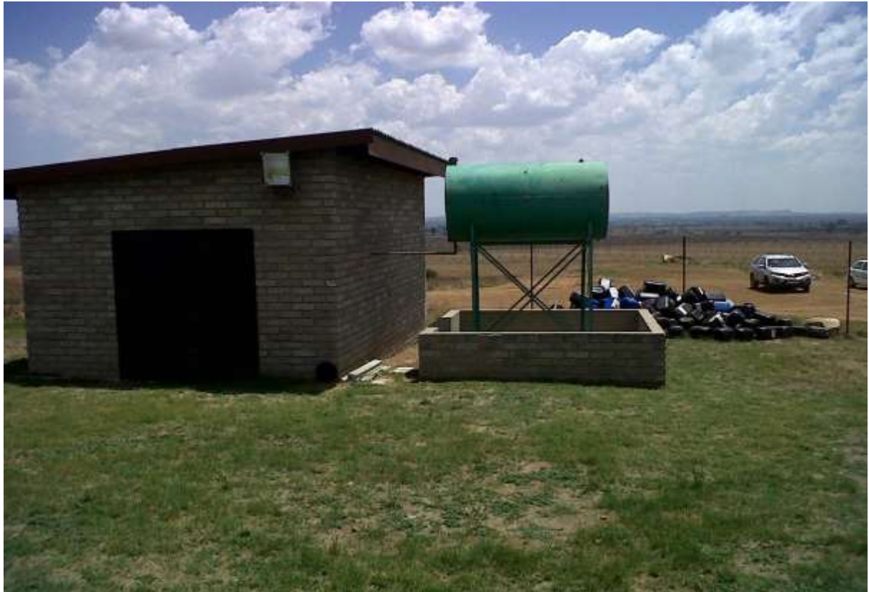
Figure 6: Backup generator and bunded diesel storage tank
