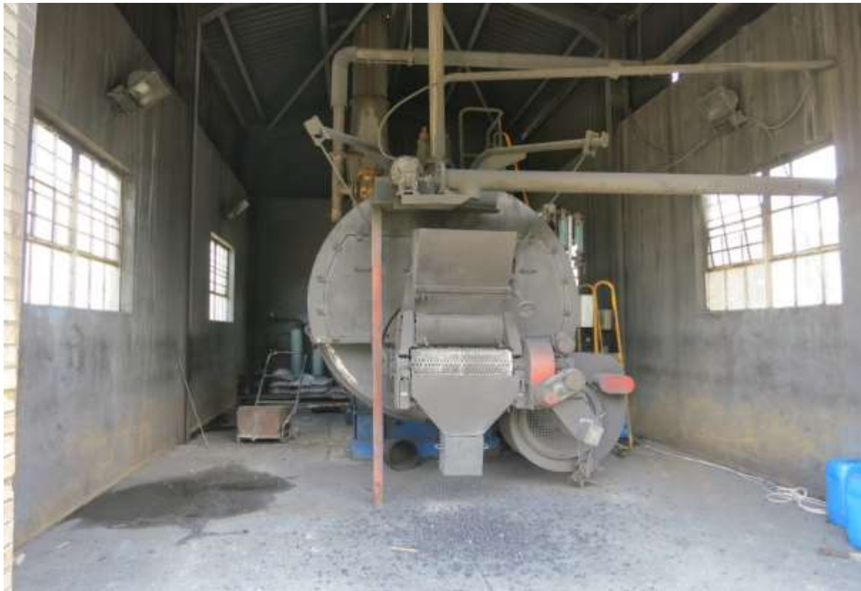
Figure 8: One of two coal fired boilers used to generate steam on site
