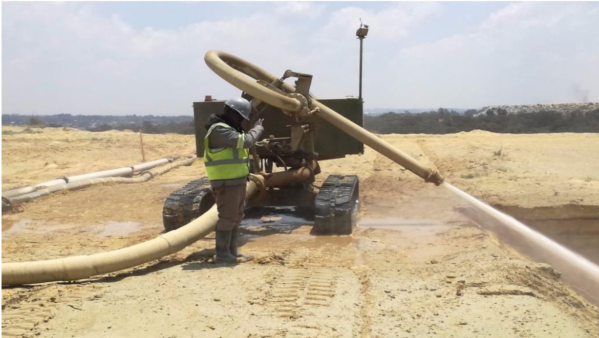
Figure 2-3: Mobile tracked hydraulic monitor on a tailings facility in South Africa
