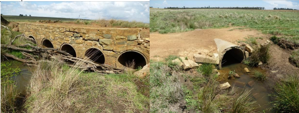
Confinement of longitudinal flow resulting in scouring (right) and channel incision (left)
