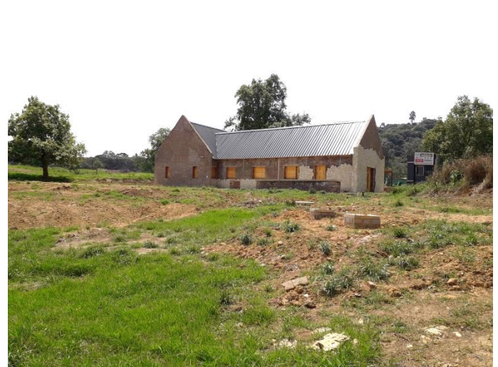
Figure 3: 'Cowshed' built on the footprint of the original. Application had to be made to AMAFA for its demolition because there were no foundations.
