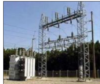
Figure 5-3: Example of a transformer, incoming power from the transmission grid, a set of switches for the incoming power and distribution bus plus three voltage regulators.
