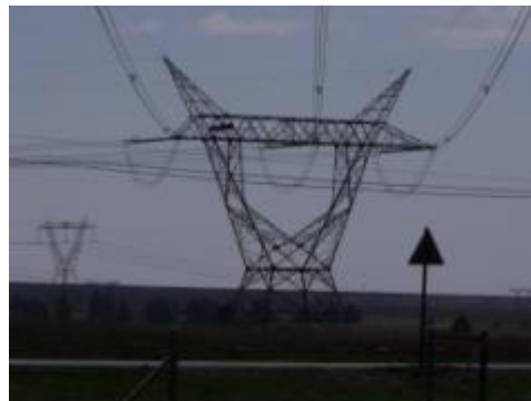
Figure 1-3: Example of 400 kV Tower
