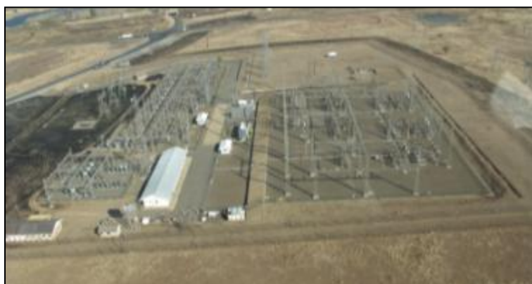
Figure 1-4: Example of a substation
