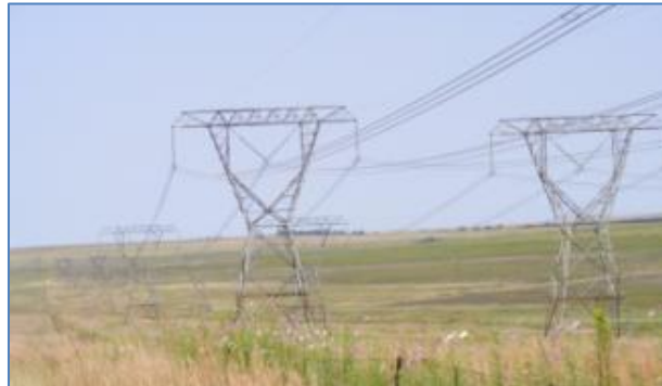
Figure 5-2: Typical transmission power lines.
