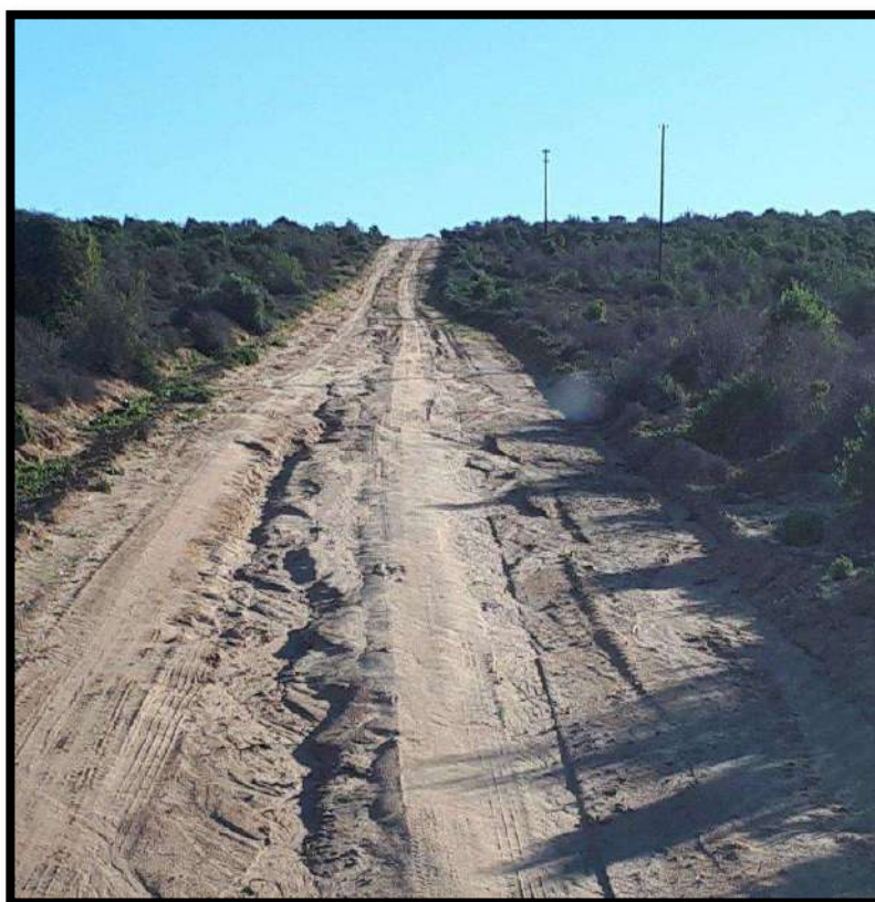
Figure 1-8: Note the erosion damage along the main farm access roads with sandy soil condition, running on relative steep gradients.
