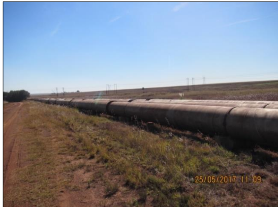
Figure 9: View of road and pipeline running along Low-level Water Return Dam servitude
