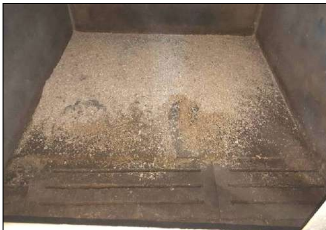
Photo 7.1: Photographic view of the concrete floor and flush channel system at the existing GTC facility.
