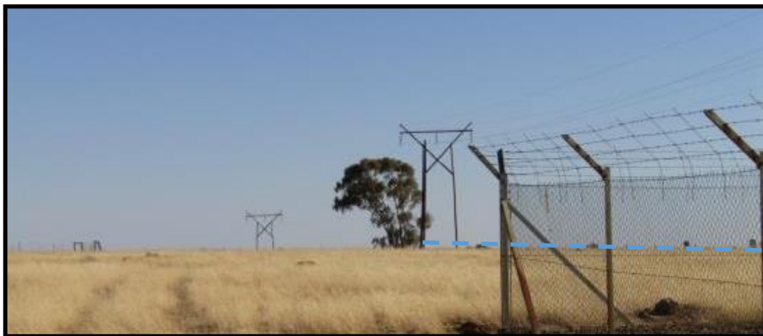
Photo 10: View of the Powerline Route from Rouxville Substation
