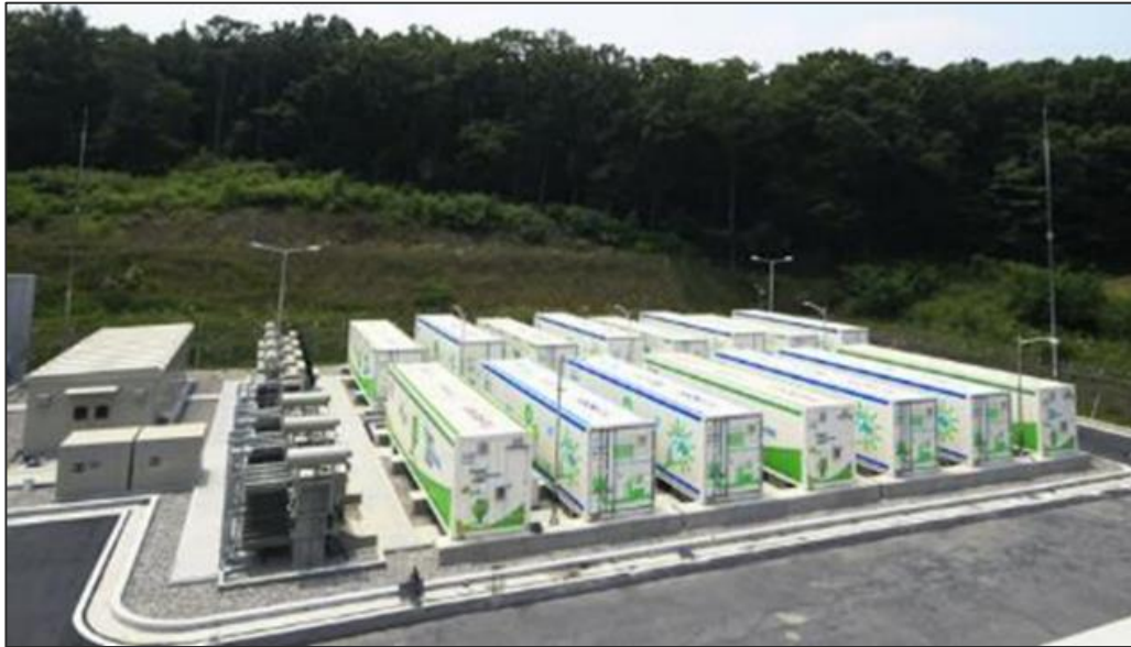
Figure 4-4: Example of a Lithium-Ion BESS installation
