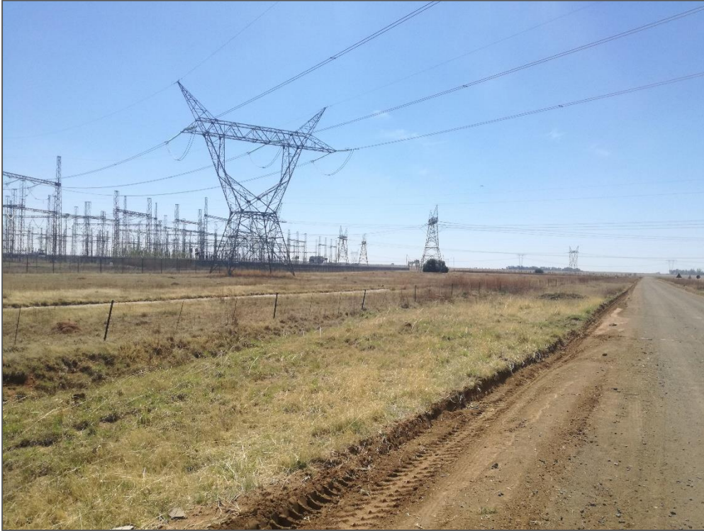
Figure 7-49: High voltage power lines feeding into Perseus Substation.
