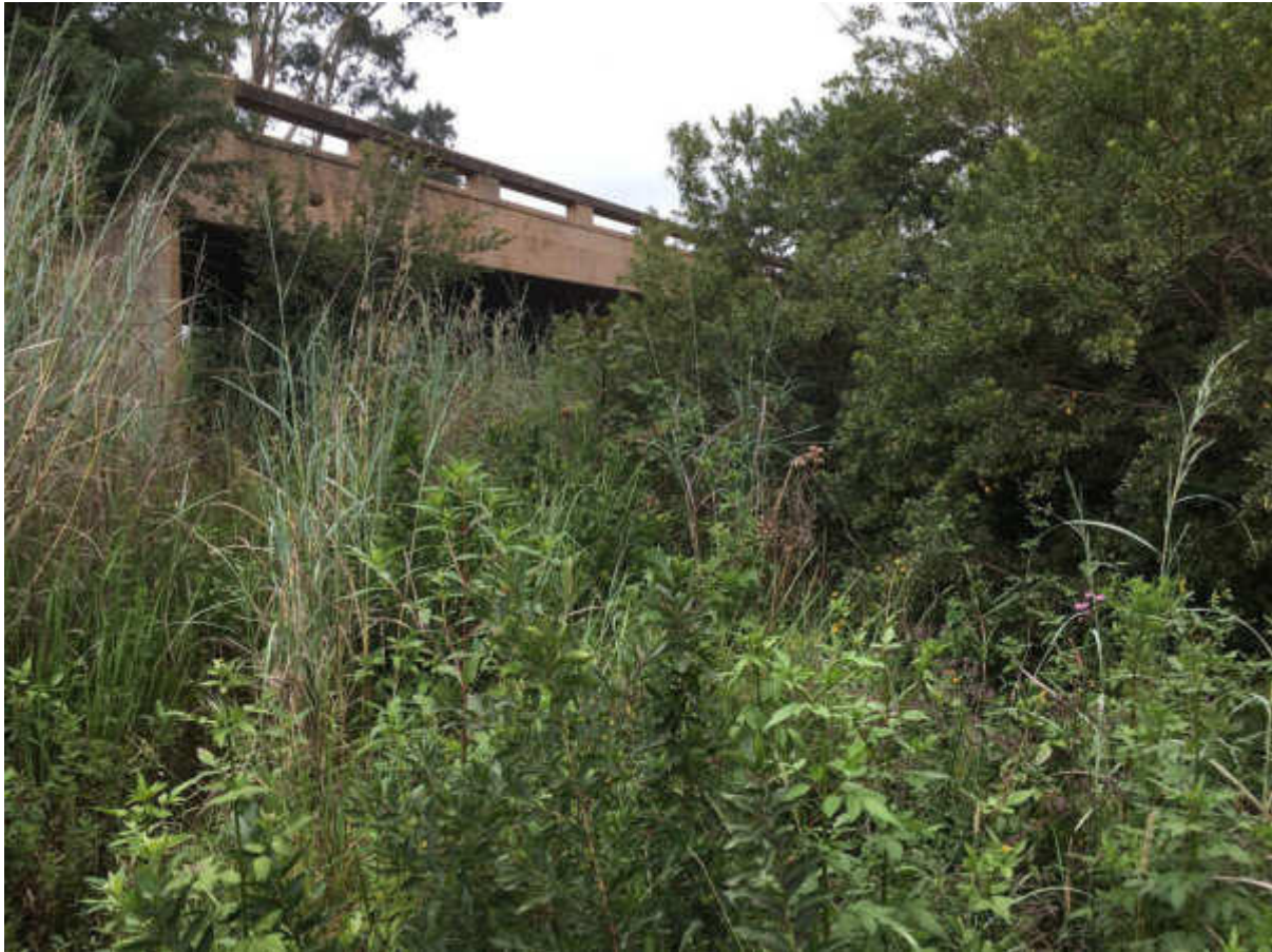
Figure 5: The bridge crossing on the M10 where the electrical line will cross (on the western section).
