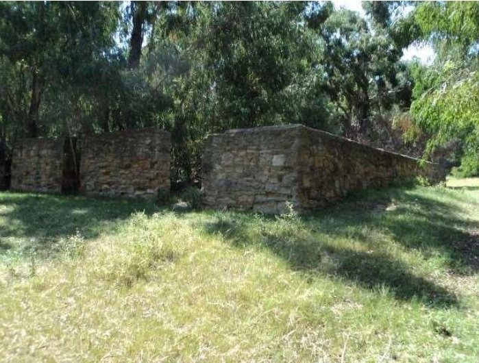
Figure 30: Example of a dilapidated historical kraal.
