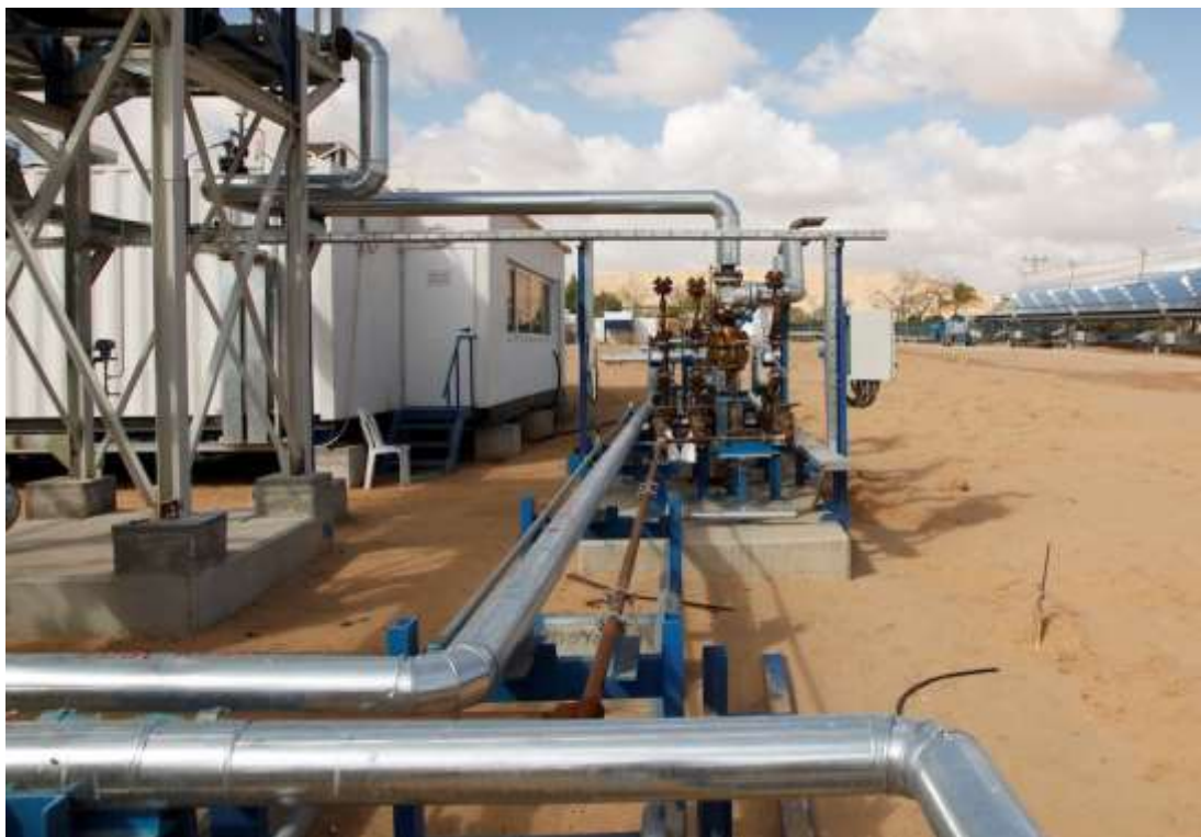
Figure 3.3: Photograph illustrating the pipes conveying the superheated steam from the solar field to the Energy Centre (courtesy of Brenmiller Energy).
