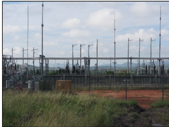
Plate 4 : Electrical substation to the north-east of the study area.
