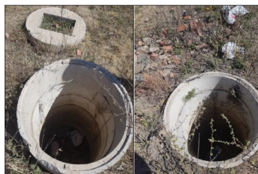
FIGURE 23: PHOTOGRAPHS SHOWING MULTIPLE MANHOLES THAT WERE RECORDED (CS5) WEST OF THE PROPOSED SITE.
