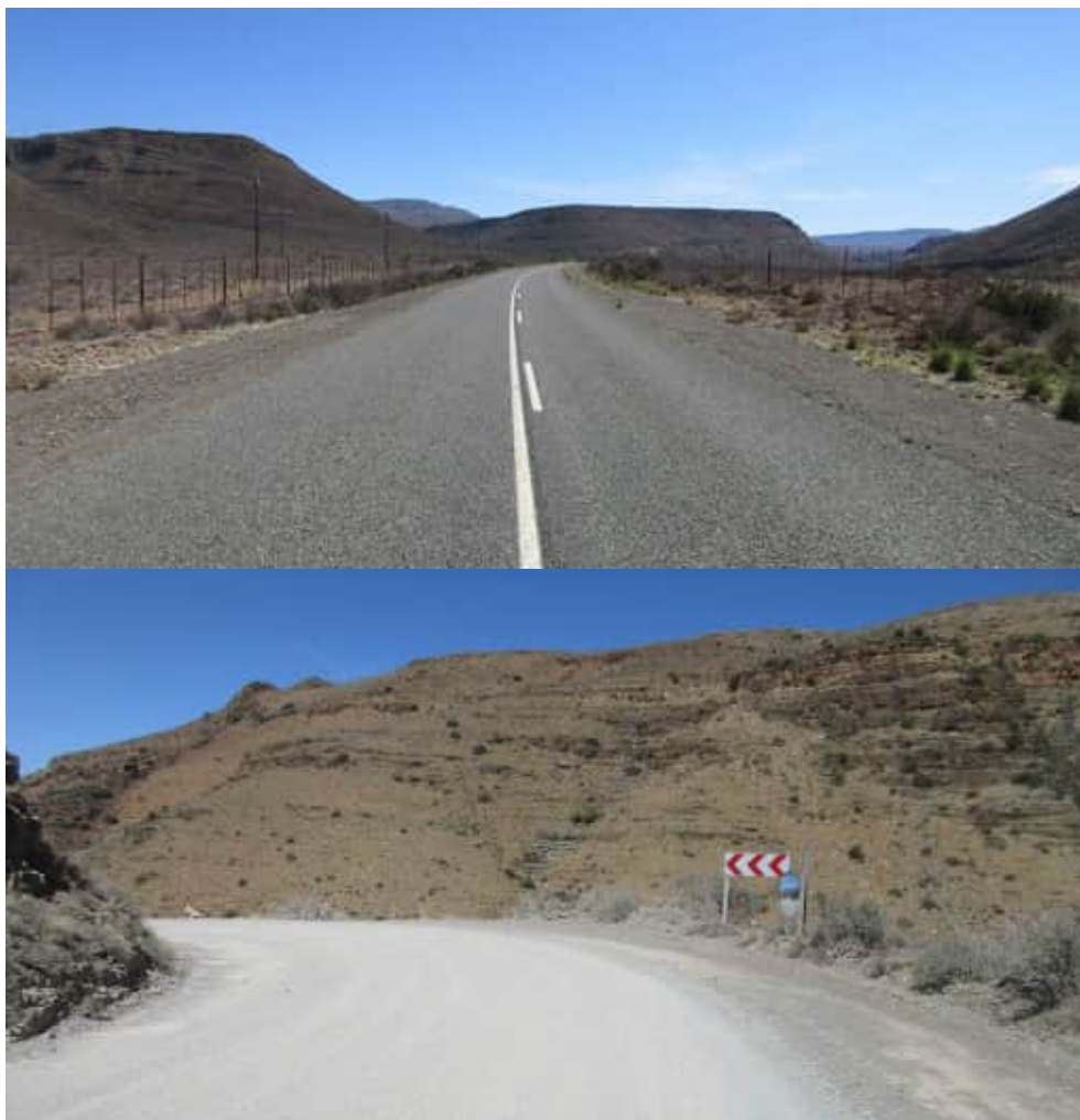
Figure 7-124: Paved and gravel sections of the R381 which will provide the main access to the site via Beaufort West
