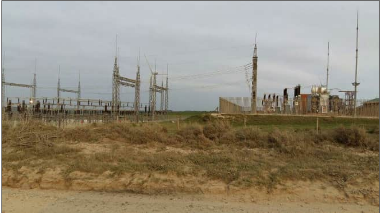
Figure 2-14: Example of a Wind Farm Substation (right) and adjoining Eskom Switching Station (left) on the Kouga Wind Farm
