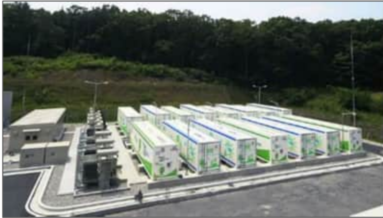
Figure 2-15: Example of a Lithium-Ion BESS installation
