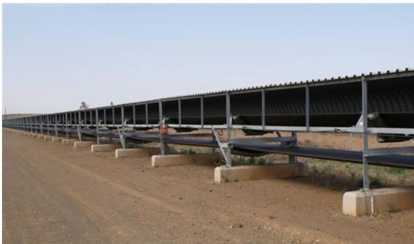
Plate 3-1: Example of typical coal conveyor from the side
