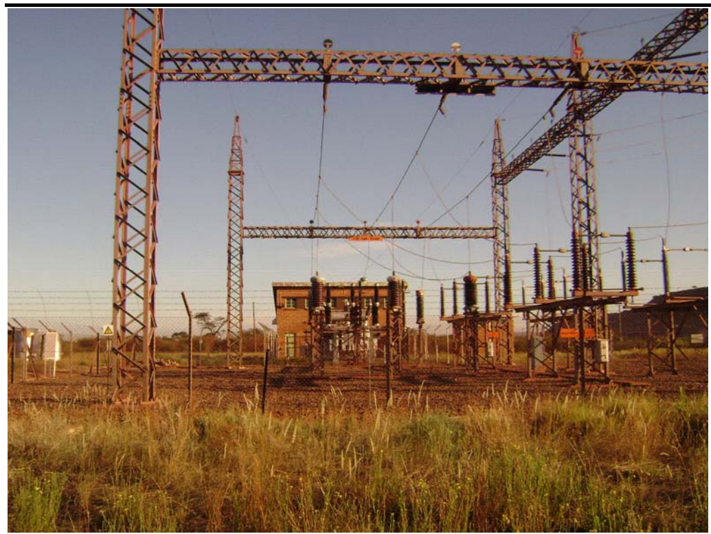
Figure 4.5 Eskom outdoor equipment (Sishen Substation)
