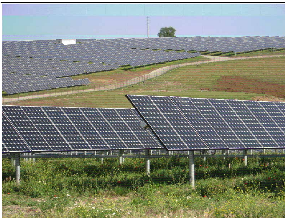
Figure 4.2 Typical PV Array
