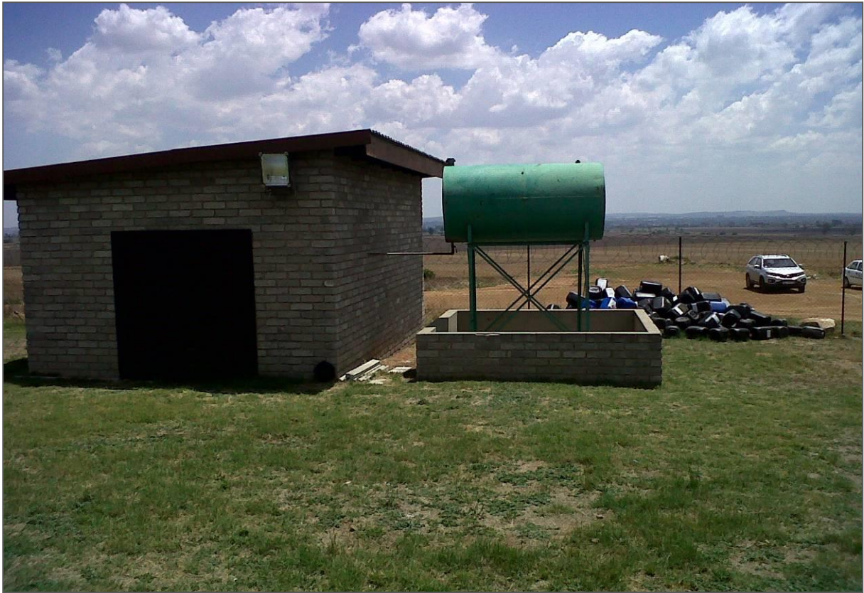
Figure 5: Backup generator and bunded diesel storage tank
