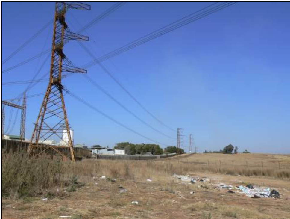
FIGURE 7: Open land and existing power lines (route 4) between Chloorkop and North Rand substations
