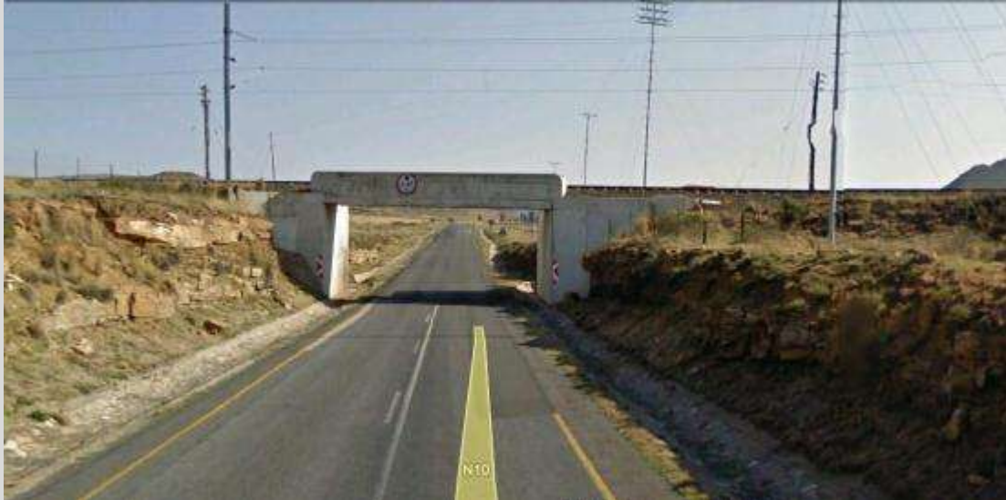
Figure 5.1. Photo of the Flonkers rail over road bridge that will be upgraded.
