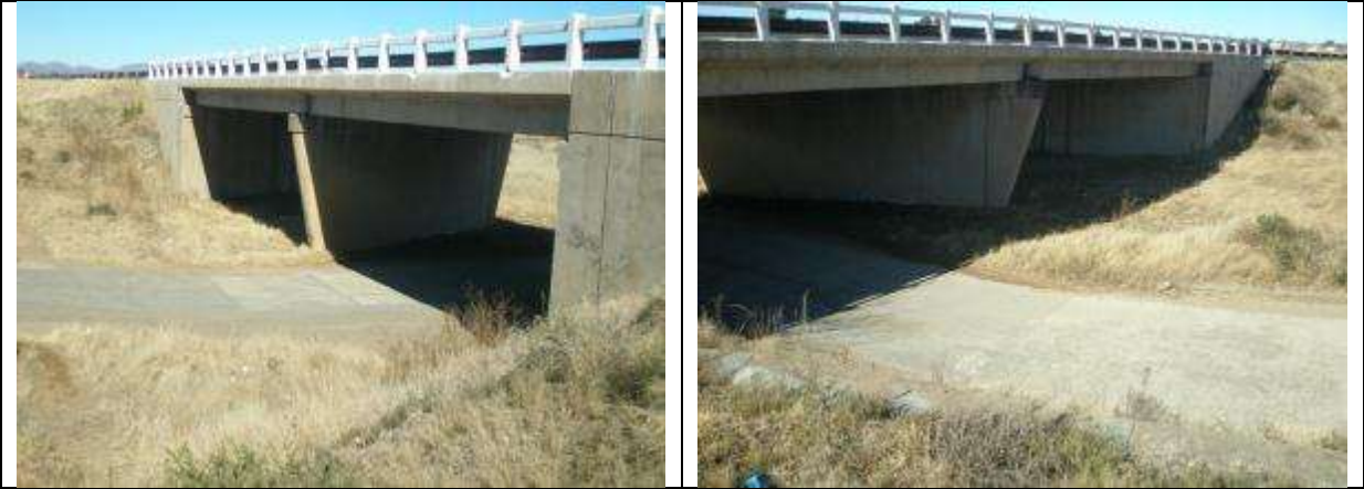
Droe River bridge: Upgrading involves a new wearing course, service/replace joint seals, and replacing balustrades with standard SANRAL detail.
