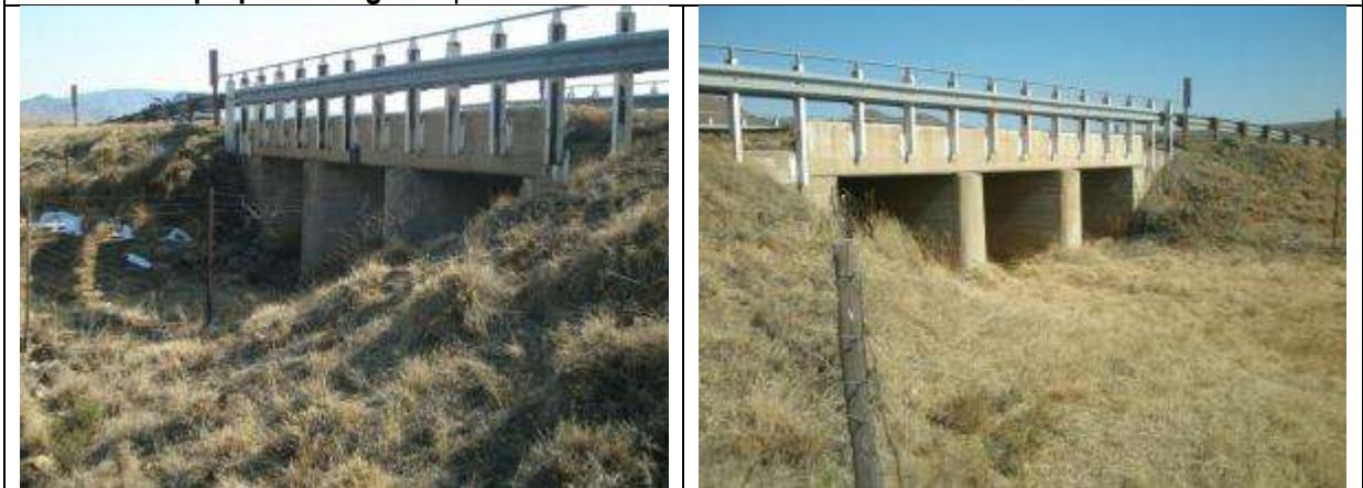
3 rd Wolwekop Spruit bridge: Widen/replace the existing bridge to suit new road alignment and cross section. Capacity improvements.
