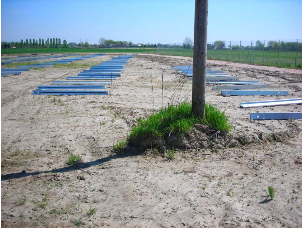
➤ Figure 9: A photo of mechanical structures for PV module support.
