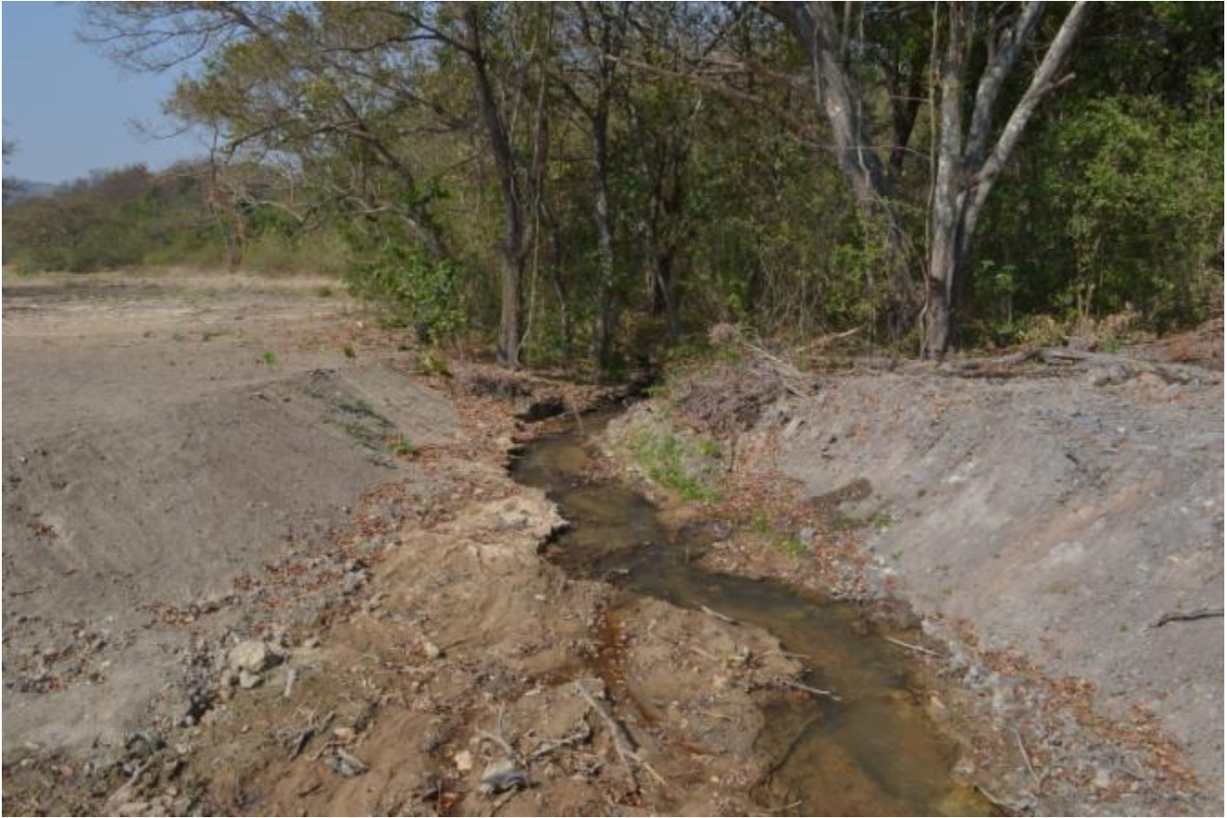
FIGURE 35: A WETLAND IMPACTED BY RECENT ROAD CONSTRUCTION ACTIVITIES ALONG THE PORTION OF THE EXISTING SERVITUDE THAT WOULD LINK THE P166 WITH THE R40 TO THE NORTH OF THE RIVERSIDE MALL AND N4 BYPASS IN MBOMBELA
