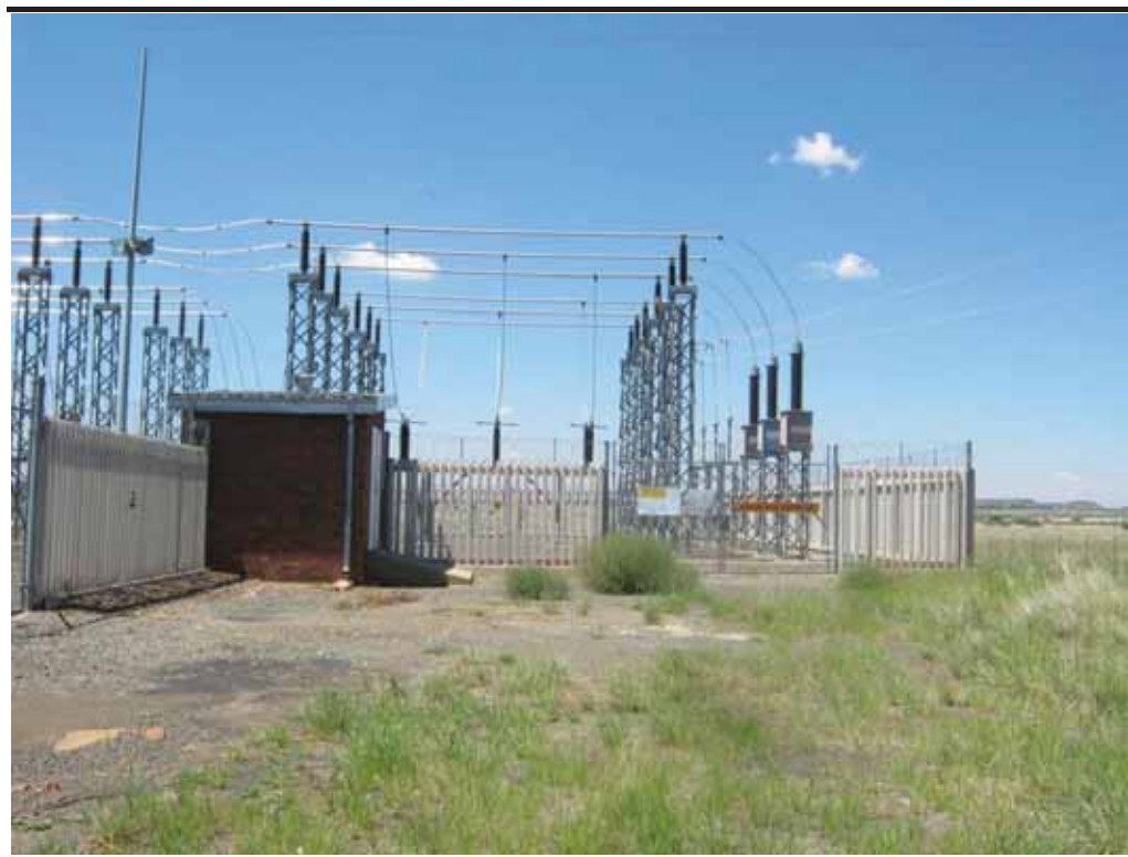
Figure 4.11 Existing Graspan Traction Substation
