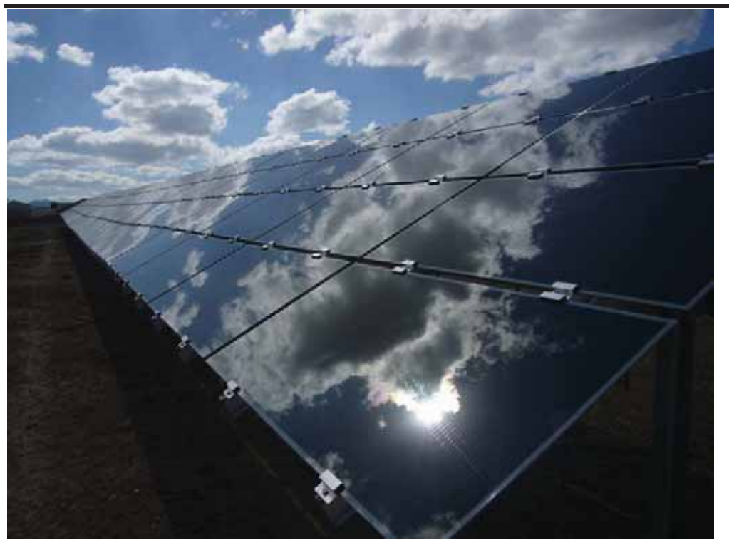
Figure 4.5 Typical PV Array
