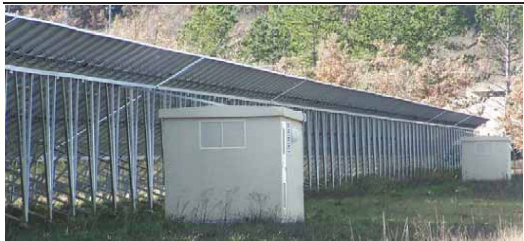
Figure 4.8 Typical Inverter/Transformer Enclosures
