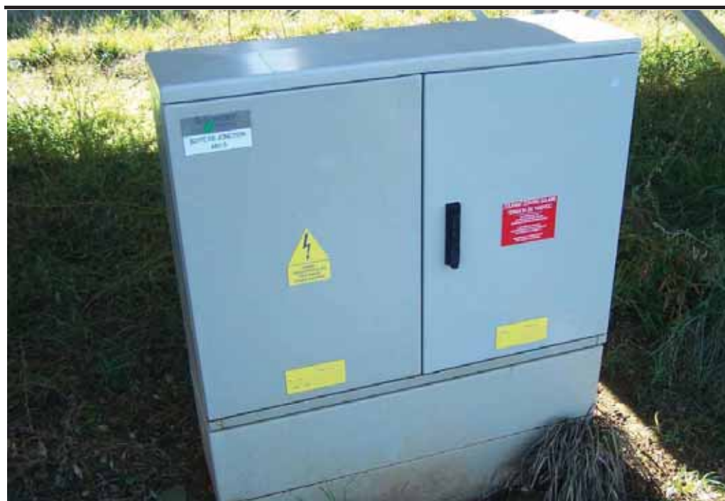
Figure 4.6 Typical Array Enclosure
