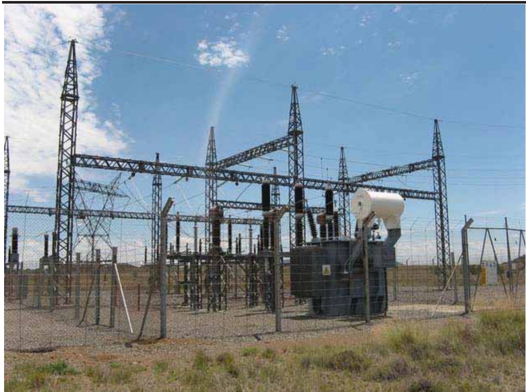
Figure 4.10 Transformer in Grid Connection Substation Yard
