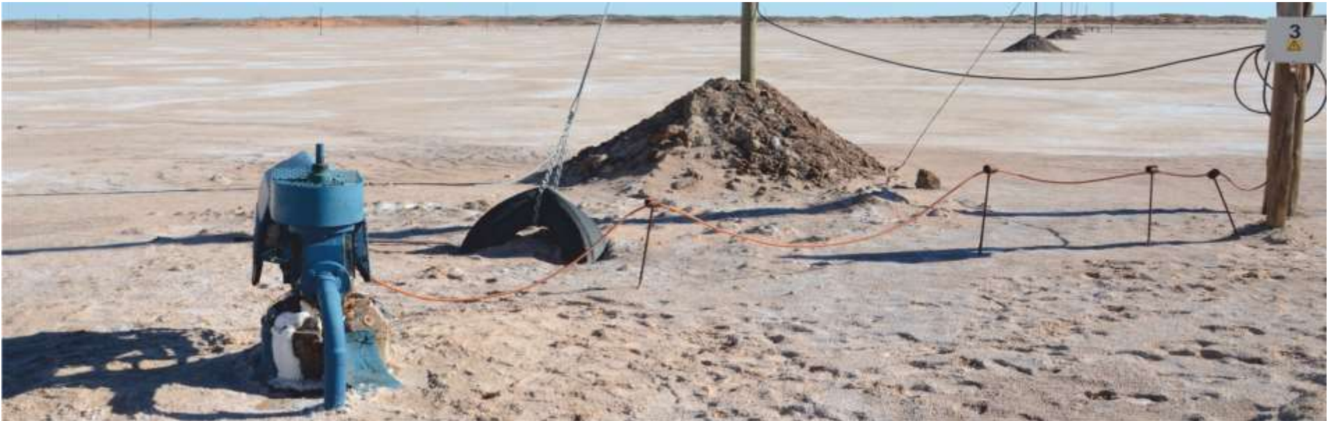
Photo 1: Typical electrically driven pump installation on pan.
