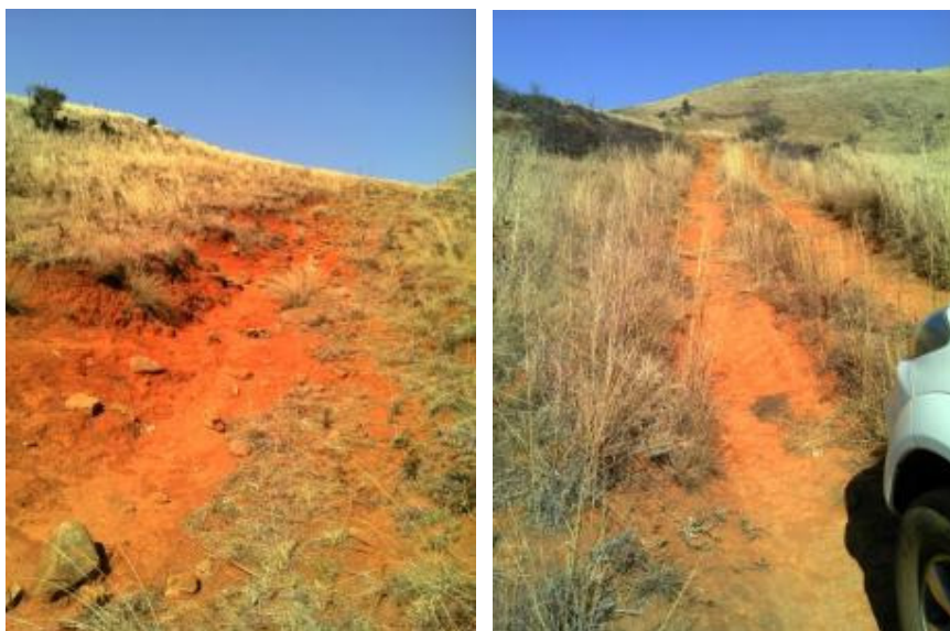
Figure 29: Deactivation of old road (left hand side photo) and protection of new road (right hand side photo) by means of gabion walls and earthen diversion berms (W42C-02-217-00)
