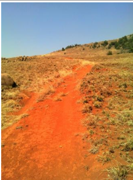
Figure 33: Surface cross drain (interventions W42C-02-227-00 and W42C-02-228-00) looking in a south and south-easterly direction
