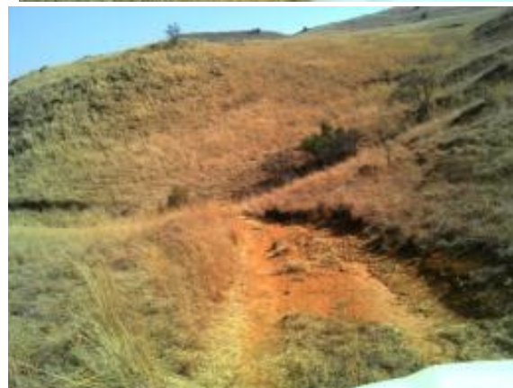
Figure 32: Surface cross drain (interventions W42C-02-221-00 to W42C-02-226-00) looking in a south and south-easterly direction
