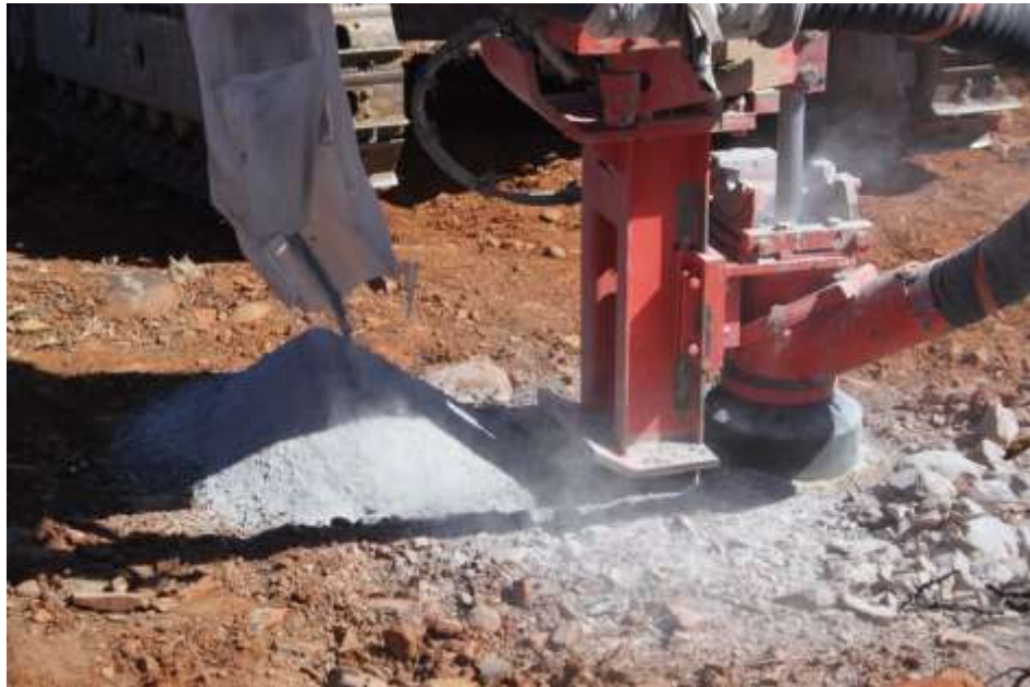
Photo 5: Dust extraction system on percussion rig and sampling point for chips
