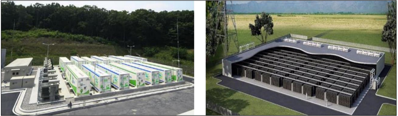
Figure 9. Battery Energy Storage System (BESS)
