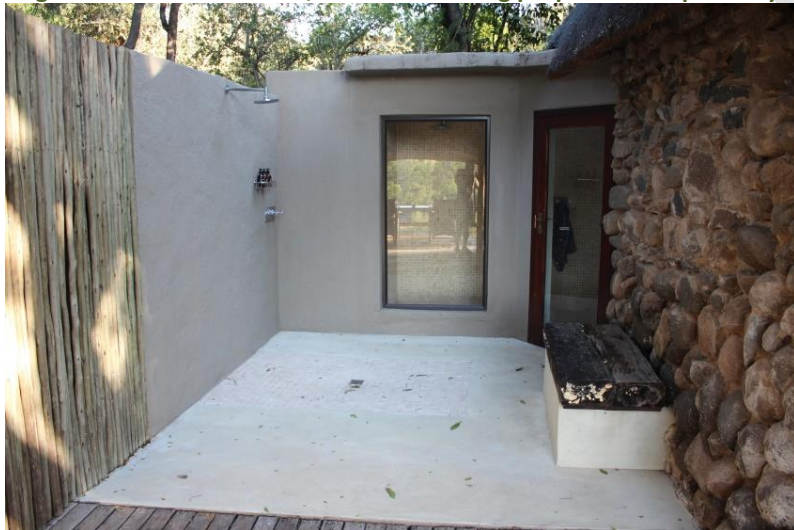
Figure 11: Room 9 outside shower which will be enclosed.
