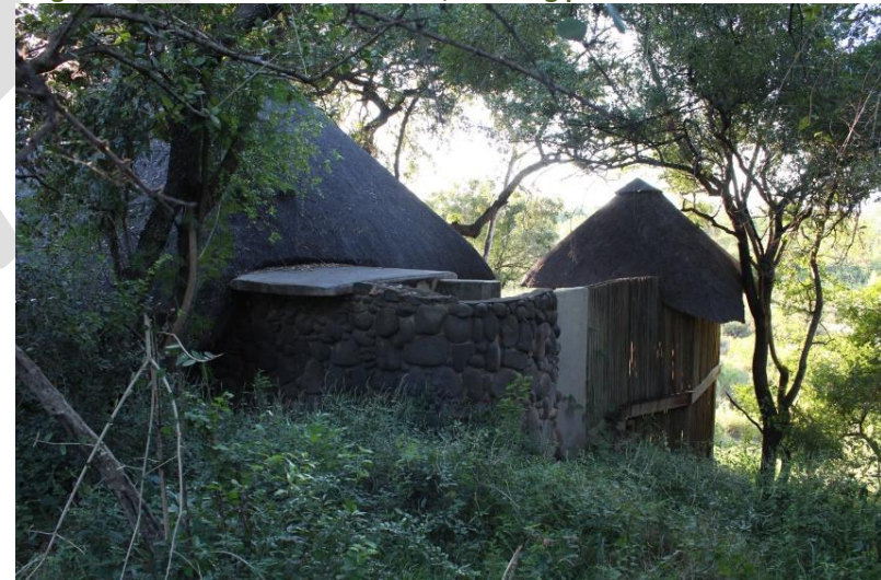
Figure 12: Room 9 outside shower which will be enclosed for a new bathroom area
