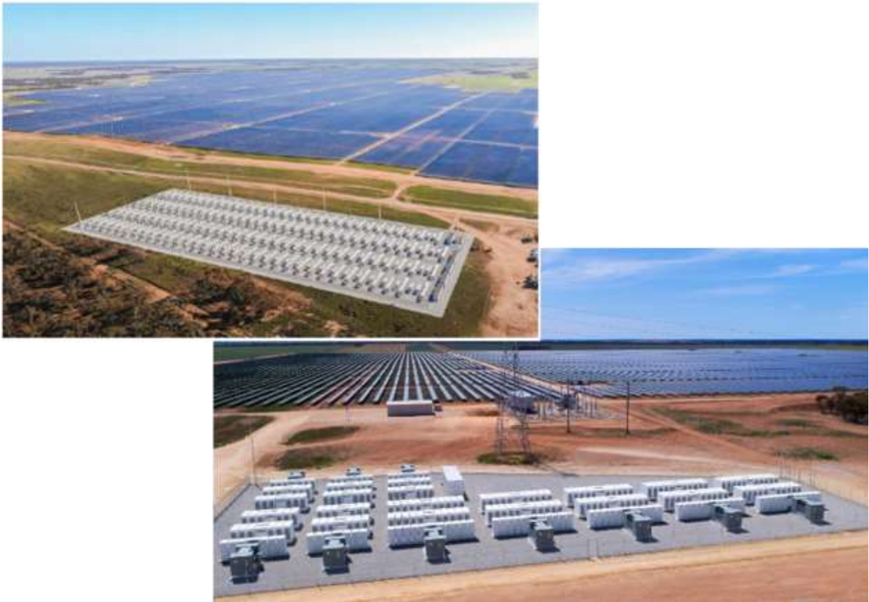
FIGURE 2.3.1.1 – Images of Typical Centralized AC Coupled BESS Systems Servicing Solar Power Farms
