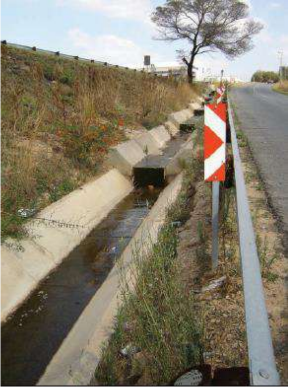
Figure 6: Stepped energy dissipater channel (AEP, 2016)
