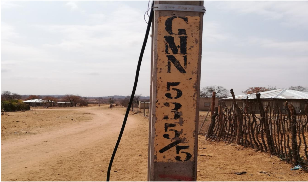
The existing pole number where they are going to connect with the proposed powerline
