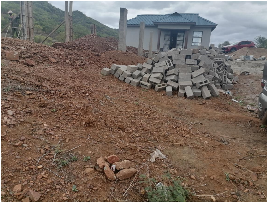
The place where transformer is required
