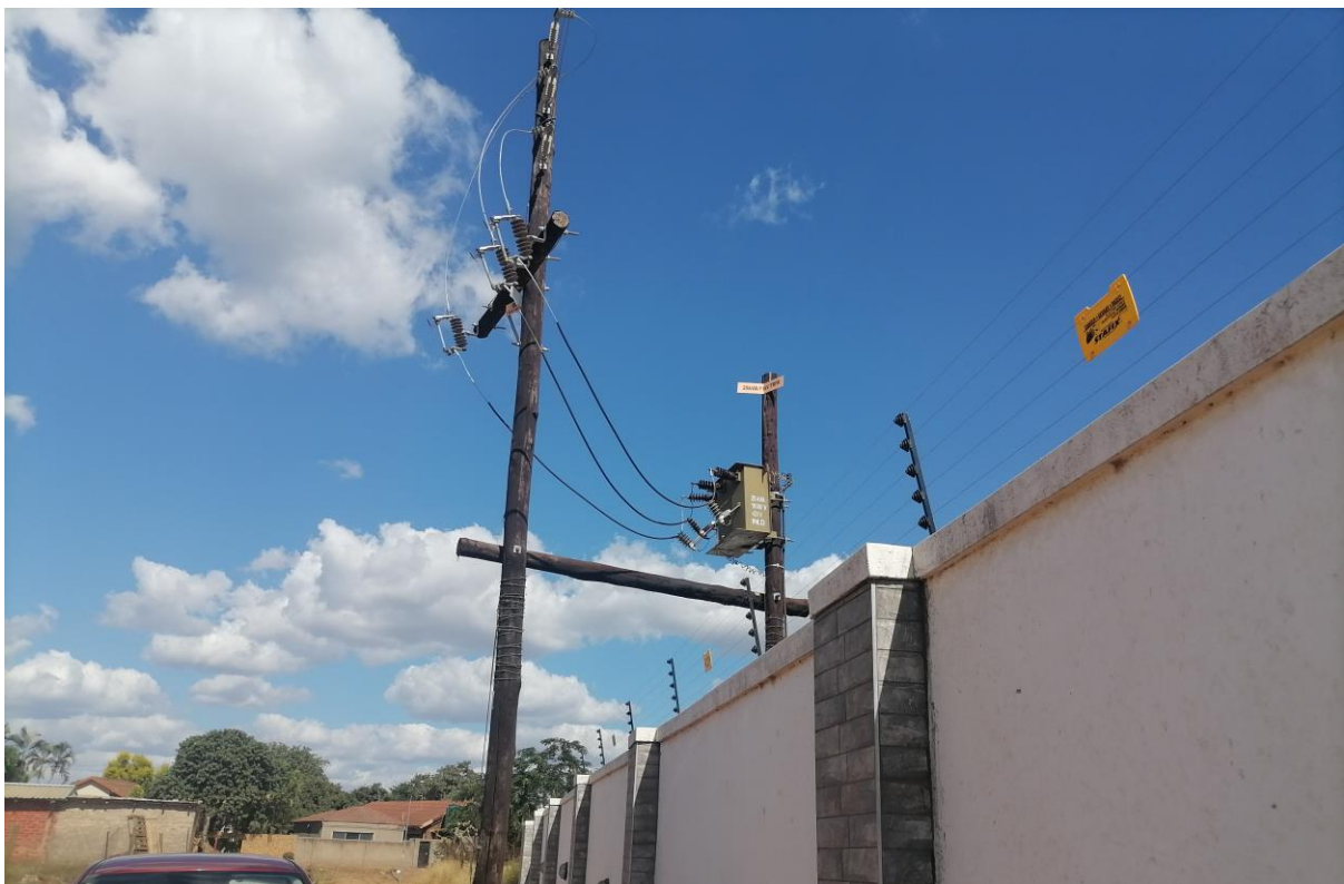
Picture showing the existing transformer on site
