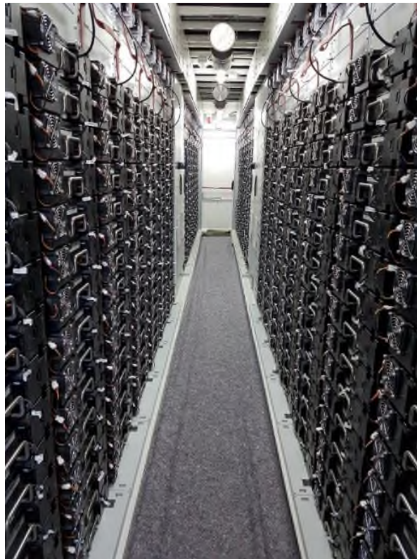
Figure 2.5: Li-Ion BESS internal design and implementation of a container used within a BESS. The image shows a series of sealed battery cell packs within a containerised module (Source: Enel Green Power).
