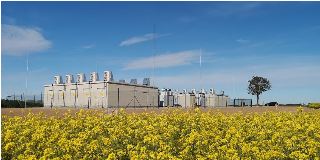
Figure 2.3: Li-Ion BESS implementation for a Renewable Energy facility (Source: Enel Green Power).
