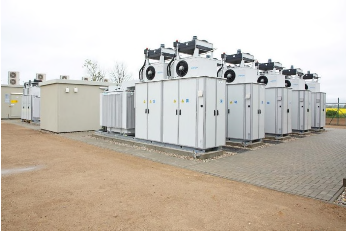
Figure 2.4: Li-Ion BESS containerised modules located within the BESS enclosure footprint (Source: Enel Green Power).
