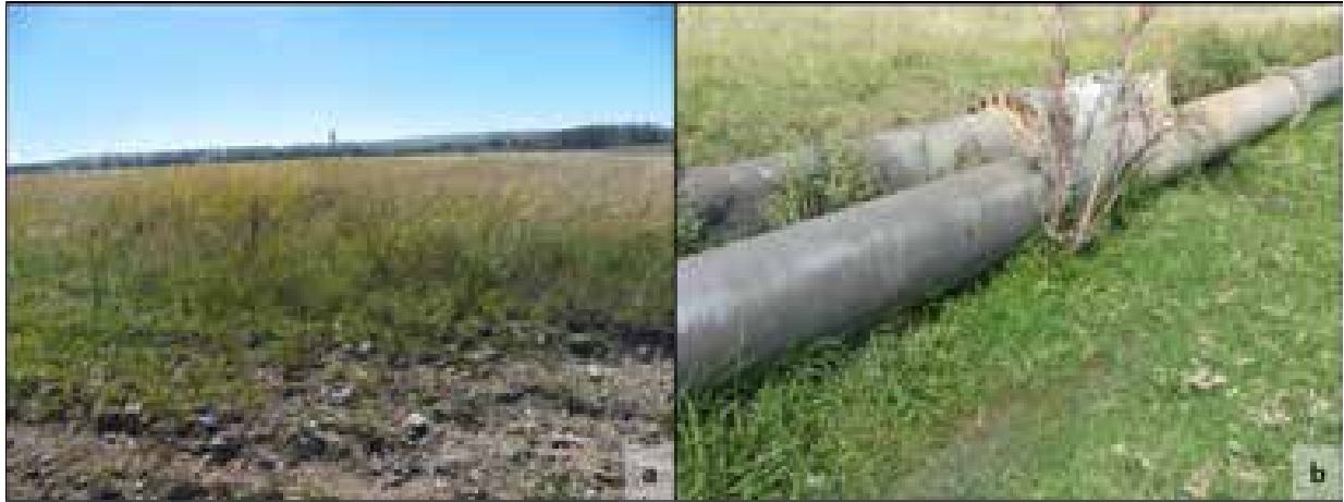
Figure 7-11: Wetland 9b (VB) photos: a) general wetland environment; and b) evidence of leaking pipe
