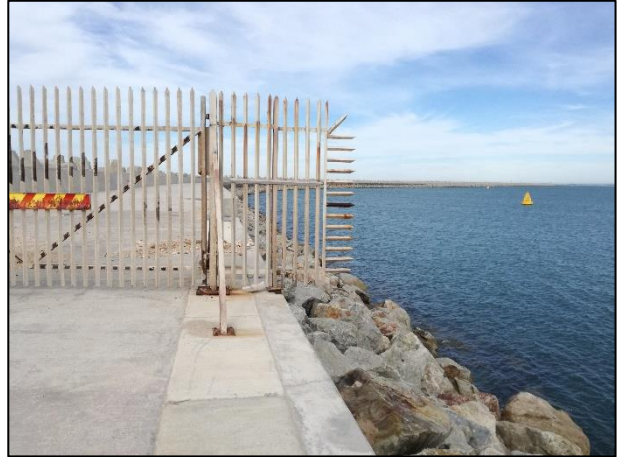
Photograph 2: View along the service corridor where the tressle supporting gas pipelines will be located
