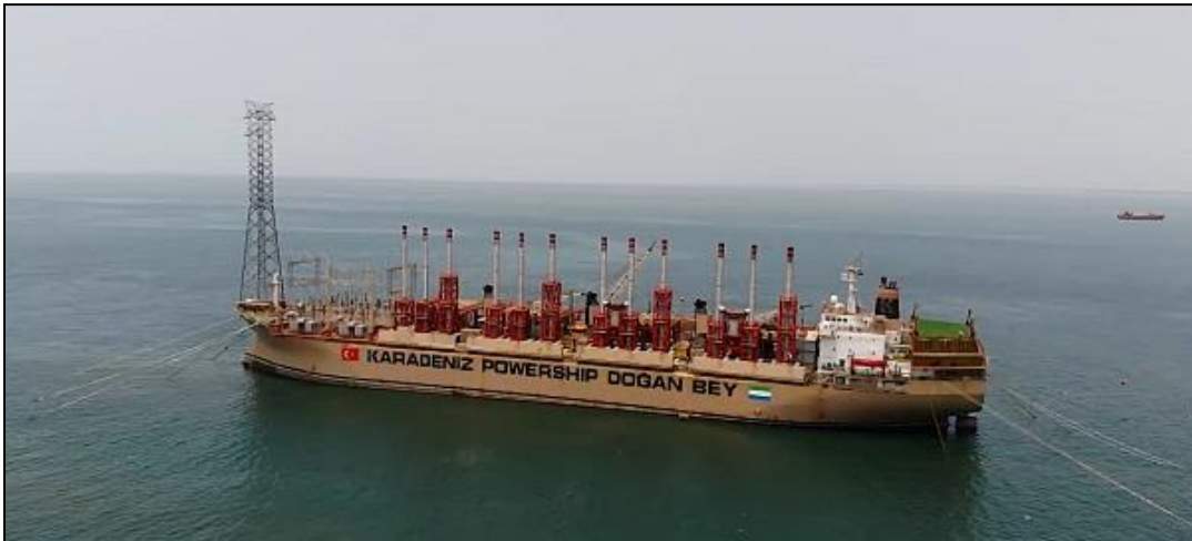
Figure 3-3: Powership mooring system.
