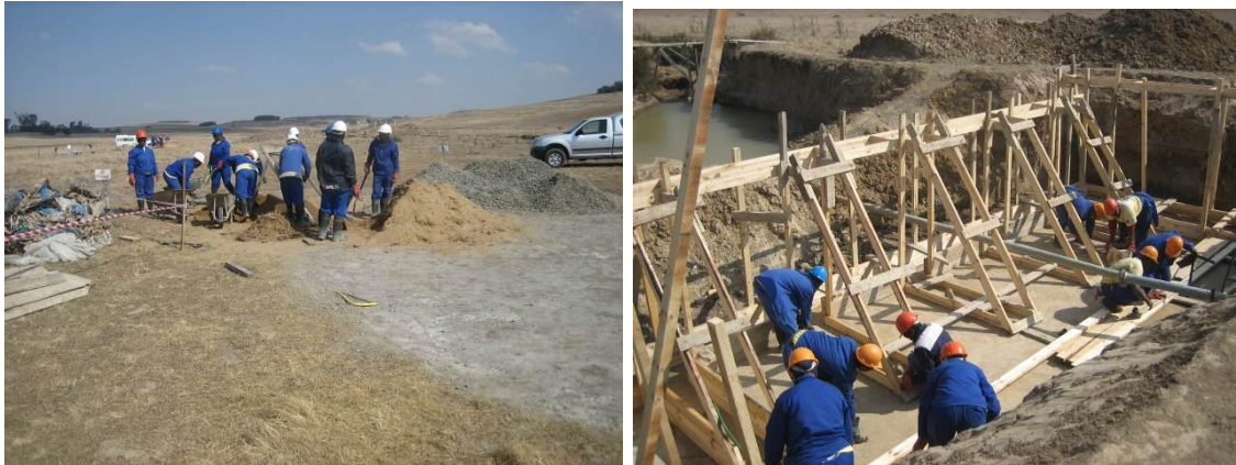
A buttress weir being built and a site being prepared by the Implementing agents
