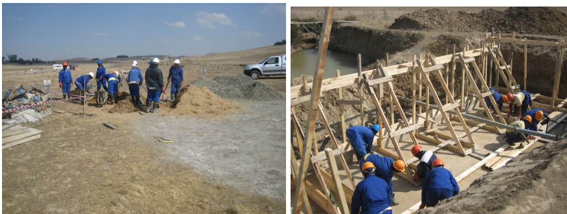
A buttress weir being built and a site being prepared by the Implementing agents
