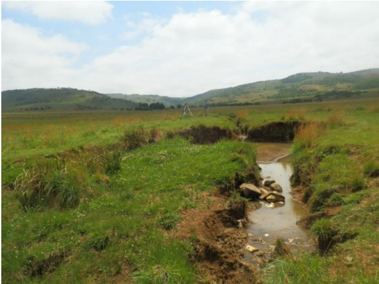
Figure 10: Photograph indication active headcut erosion to be monitored post rehabilitation on site.
