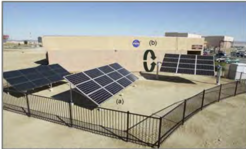
Figure 2.6: (a) Fixed axis tracking system and (b) single axis tracking system (Source: Mulilo Renewable Project Developments)
