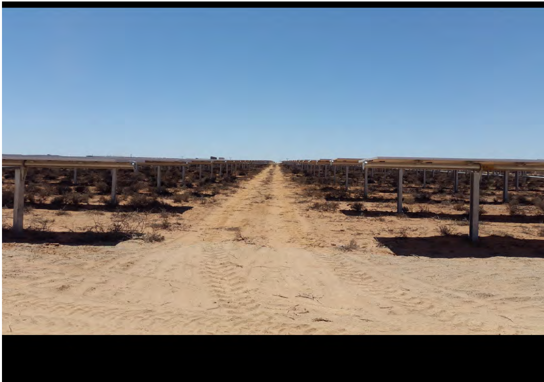
Figure 2.7: The vegetation underneath the solar panels will not be cleared, but will remain intact (Source: Mulilo Renewable Project Developments)
