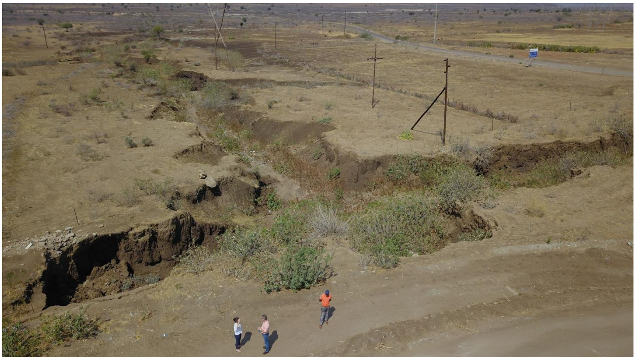
Figure 3-3: Sideways view of the existing stream crossing with severe erosion gulleys downstream.
