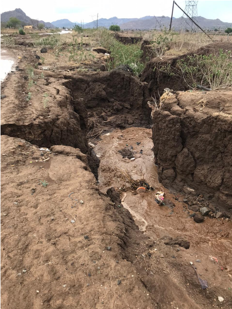
Figure D-4: Erosion dongas at outlet of Swazi Mnyamane.
