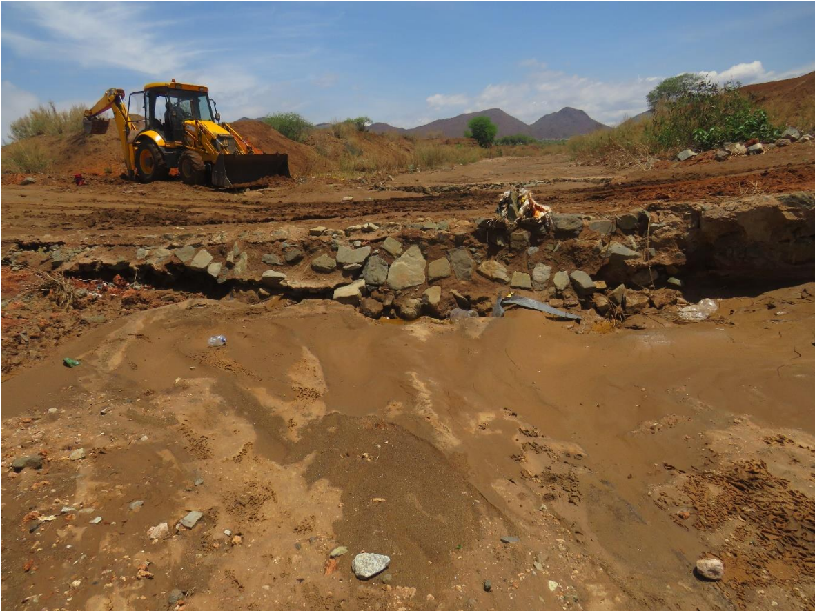
Figure D-2: Condition of Mampa stream crossing at the time of the investigation.
