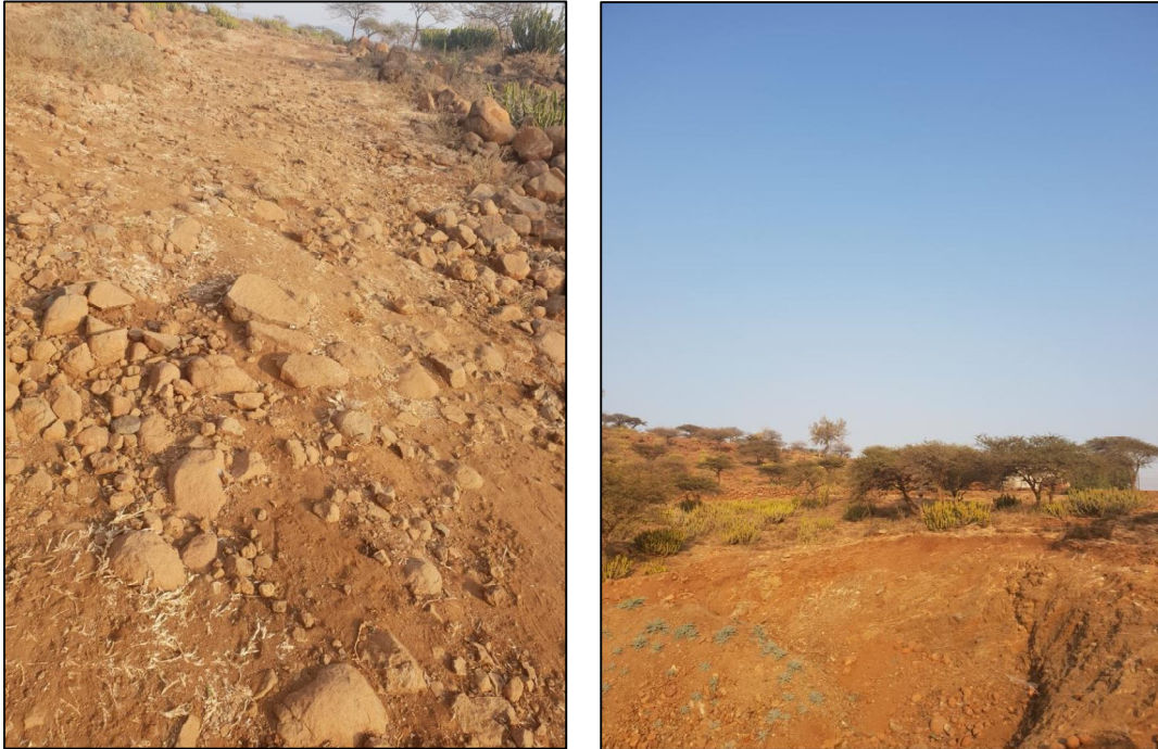
Figure 6&7: Typical conditions of sections underlain by dolerite along the proposed route.
